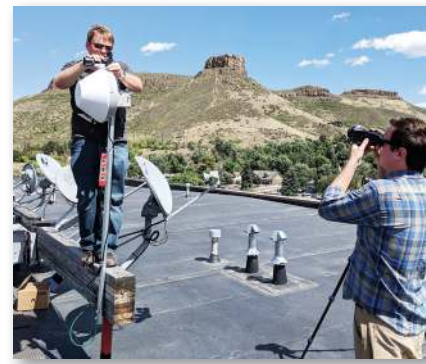
Two Au Wireless technicians install equipment on the Gateway Station condos building in Golden in July 2018.
